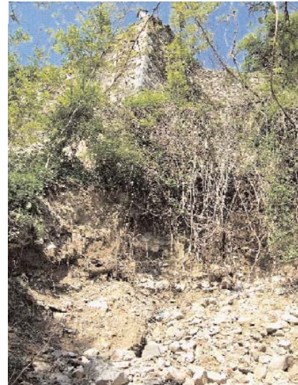
Fig. 17 Erosion at the outer wall of the Fortress.
