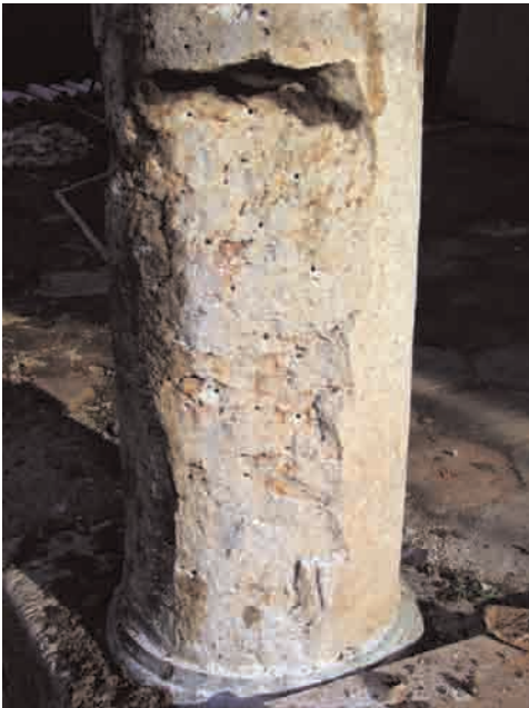
Damages on portico column
