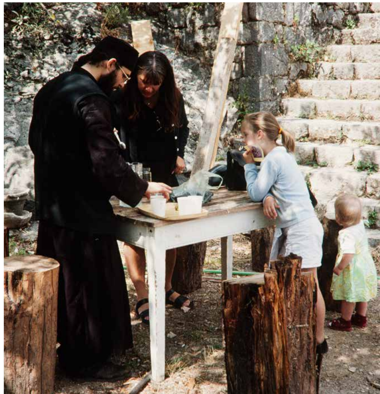
Restoration of the monastery church in Zavala, Bosnia and Herzegovina. The work has aroused a lot of interest and the monastery attracts visitors from other parts of the Balkans.
